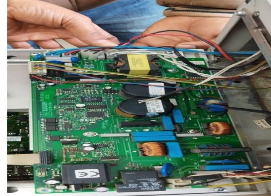
Power Supply of Inverter
